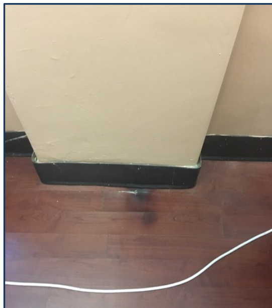
Figure A.2. Discolored floor tile in room 113 Source: VA OIG, June 4, 2019
